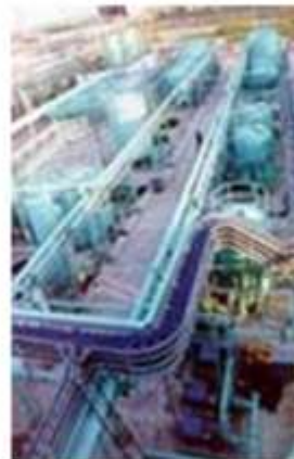
Demineralisation plant for refinery
